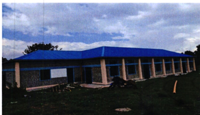
Ragia Secondary School Dinning Hall which will be used for several functions in school.
