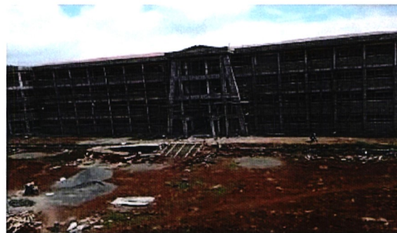
CIVIL WORKS COURT YARD RAMP AND STAIR CONSTRUCTION TO ENTRANCE BLOCK A
