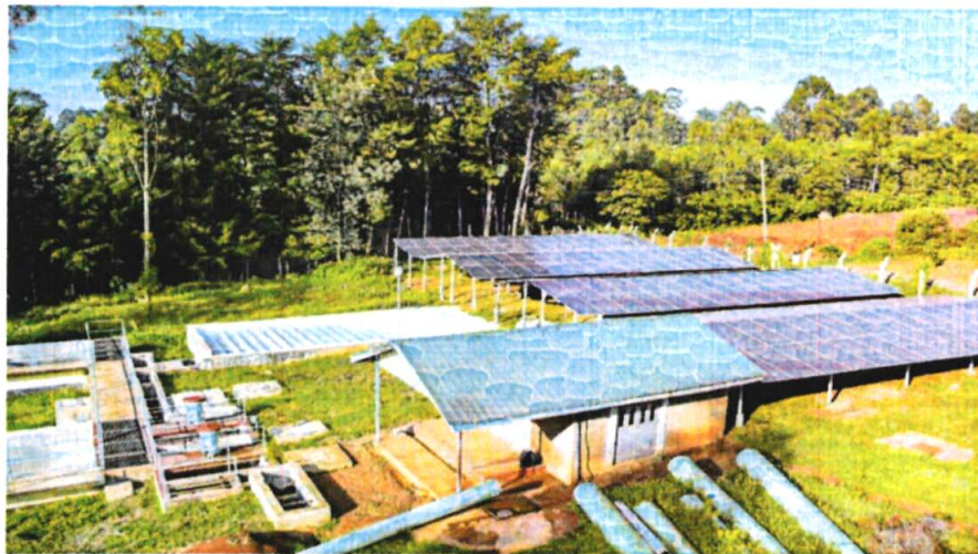
Newly installed Solar Panels at Savona Water Treatment Works (April 2025)
