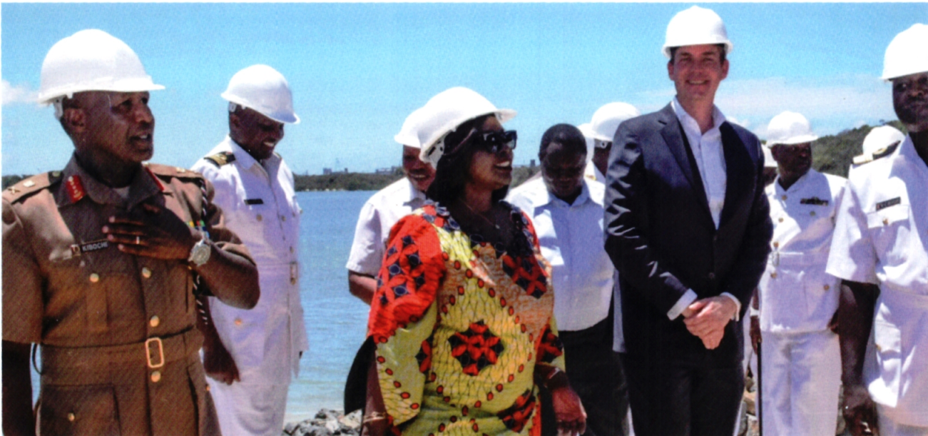
Defence Cabinet Secretary Amb Raychelle Omamo, Vice Chief of the Defence Forces Lt Gen Robert Kibochi, an official from DAMEN (a Dutch company) and senior Naval officers during the launch of the construction work of a modern Shipyard facility at the Kenya Navy Mtongwe Base.
