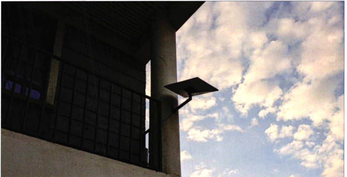
ODPP ICT staff carrying out the installation of Starlink Kits
