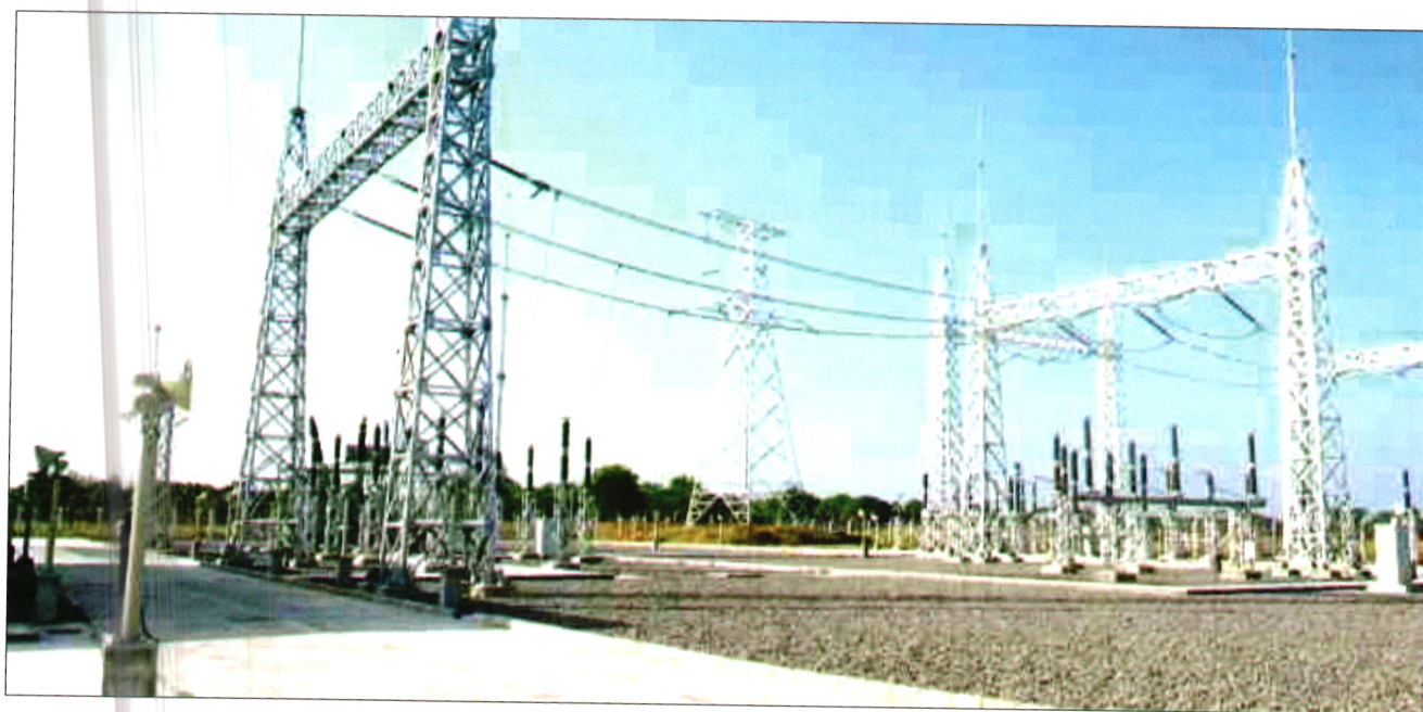
Lamu Power project
