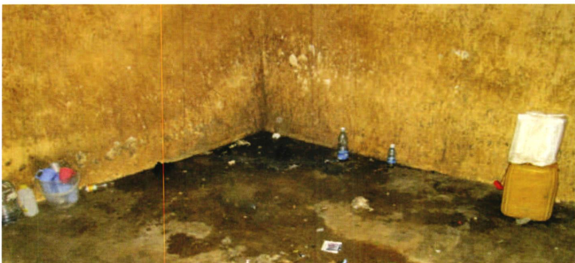
IPOA photo 2: Dirty cell at Mandera Police Station in Mandera County
