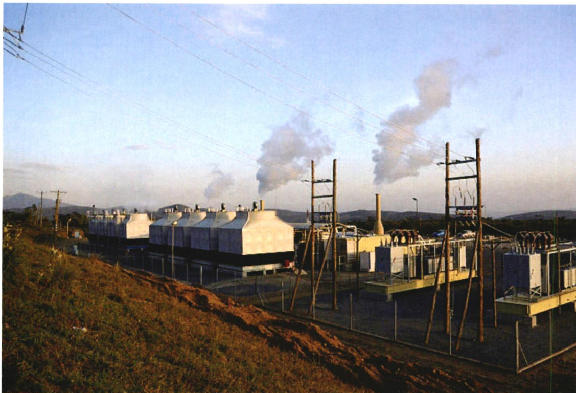
70MW Geothermal wellhead Project
