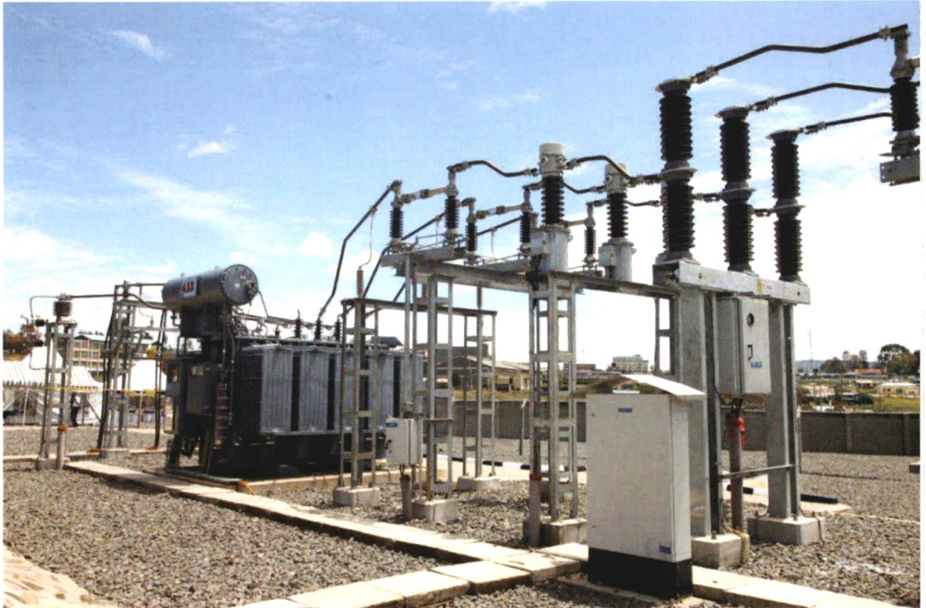
Bomet Substation during its commissioning.
