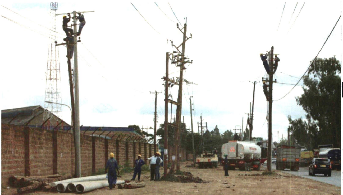
Kenya Power technicians carry out extensive work on the power infrastructure in Nairobi West as part of Operation Boresha Stima Viwandani in May 2014.
