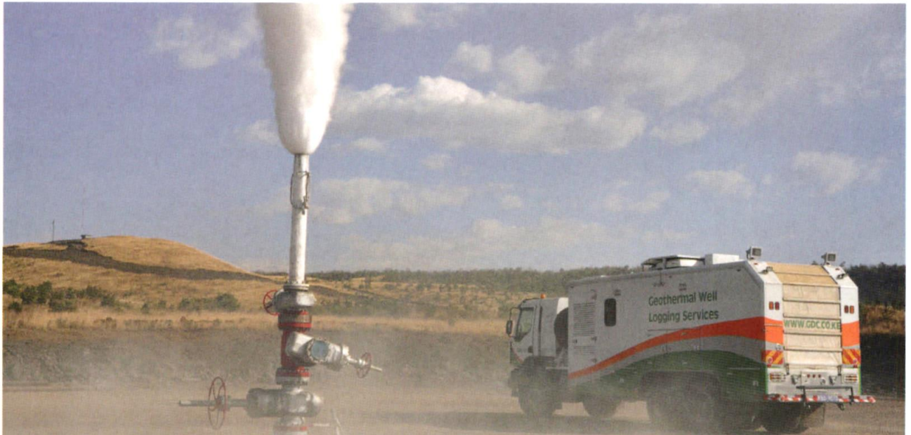
A Geothermal Well in the Menengai Geothermal Project
