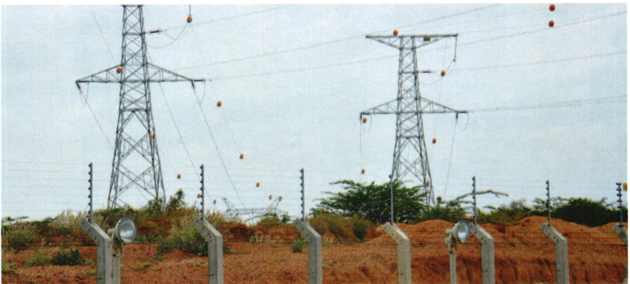
Part of the 220kV Rabai- Malindi- Garsen- Lamu Line
