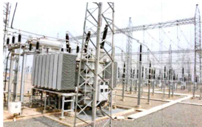
Last Mile Project, Kimuka Sub-Station in Kajiado West
