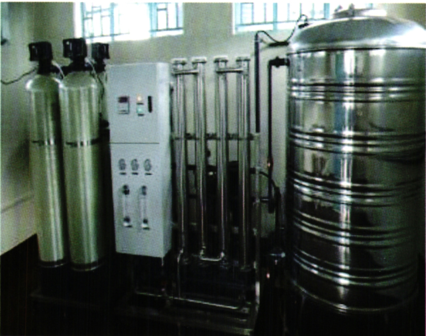
Dialysis machines and Water treatment plant at Nyeri County Referral Hospital
