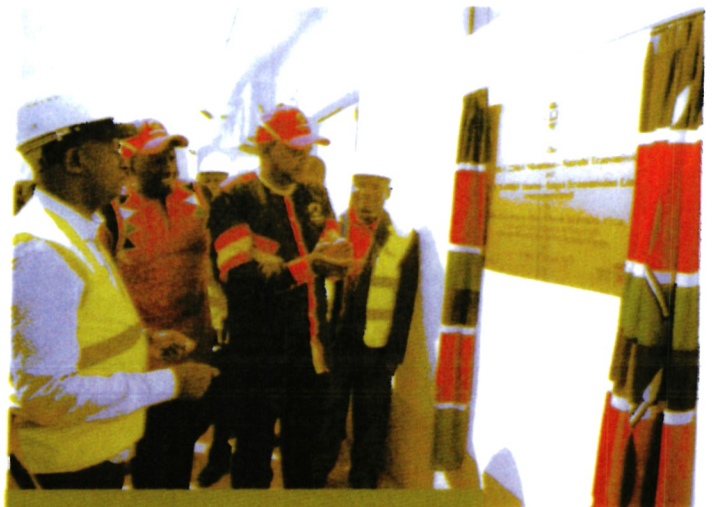
H.E Hon. Uhuru Kenyatta, C.G.H., commissioning Mambasa - Nairobi and Suswa - Isinya projects at Suswa substation
