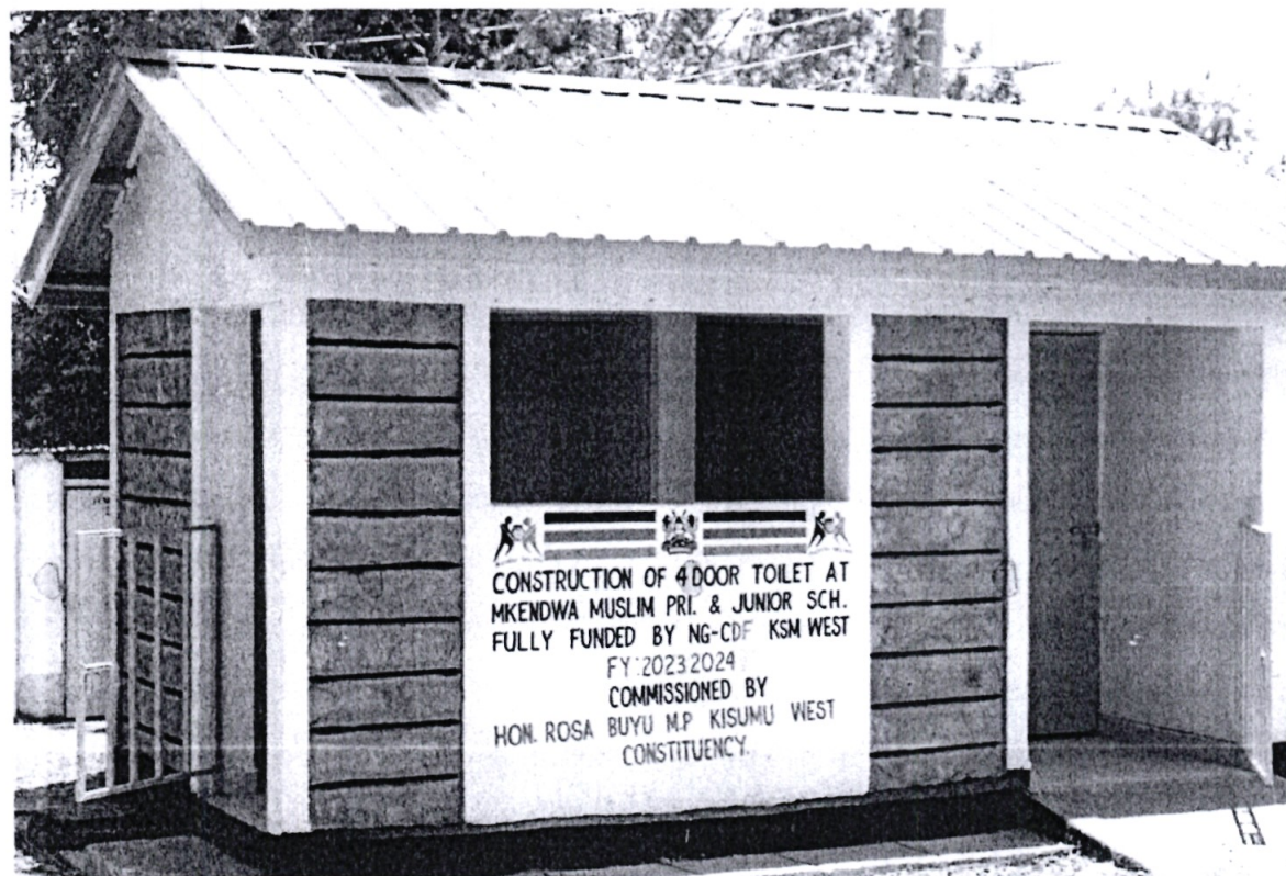
Fig 1.6: Photo of a completed construction of 4 door toilet at Mkendwa muslim primary and junior school
