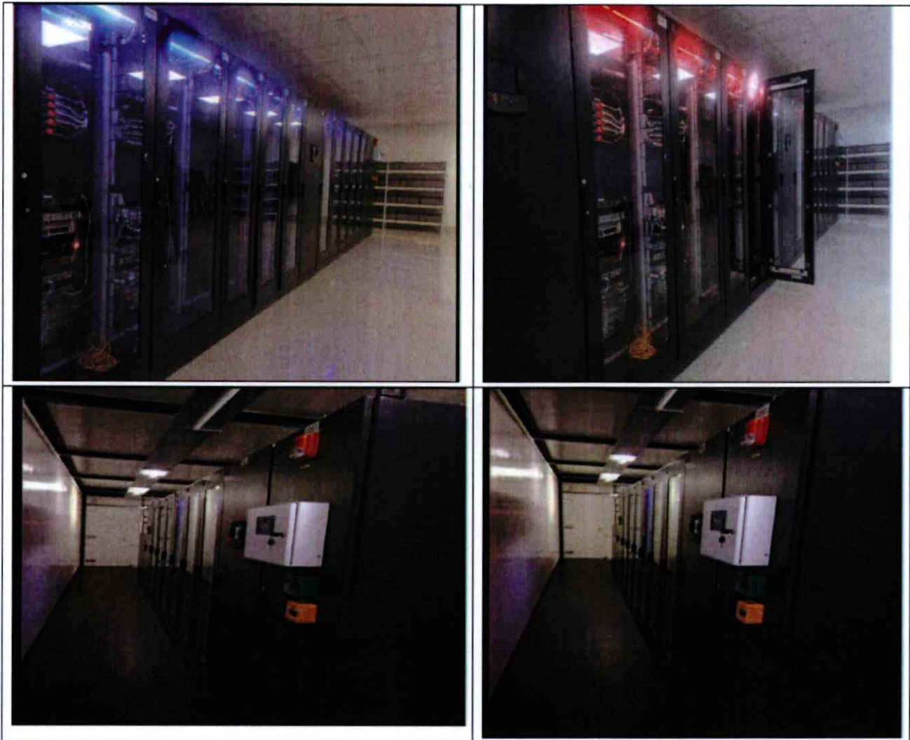
Figure 32: Data Recovery Centre
