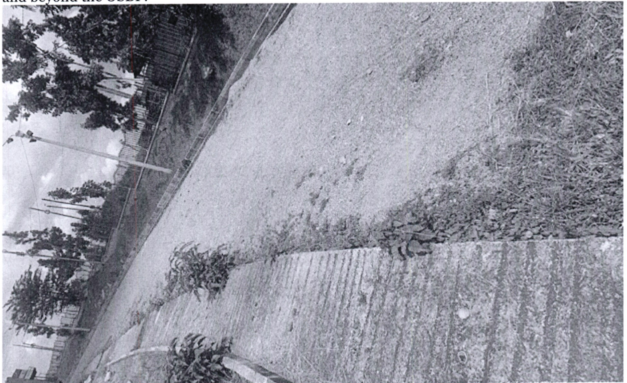
Current state of the incomplete out-bound road
