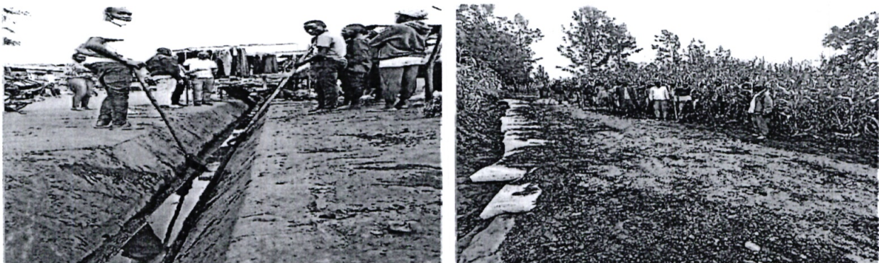
Figure 7: Manual Light grading at Ilima Ward
