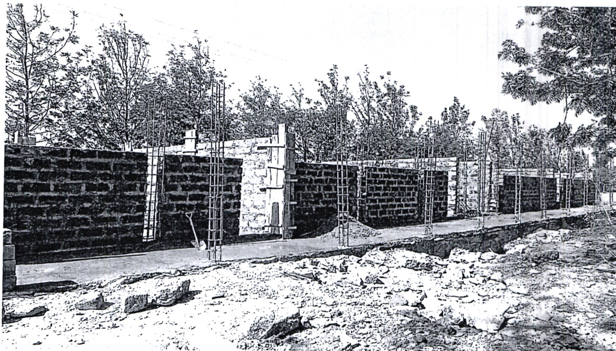
Ongoing Construction of 4No of new classroom at St John Primary School.
