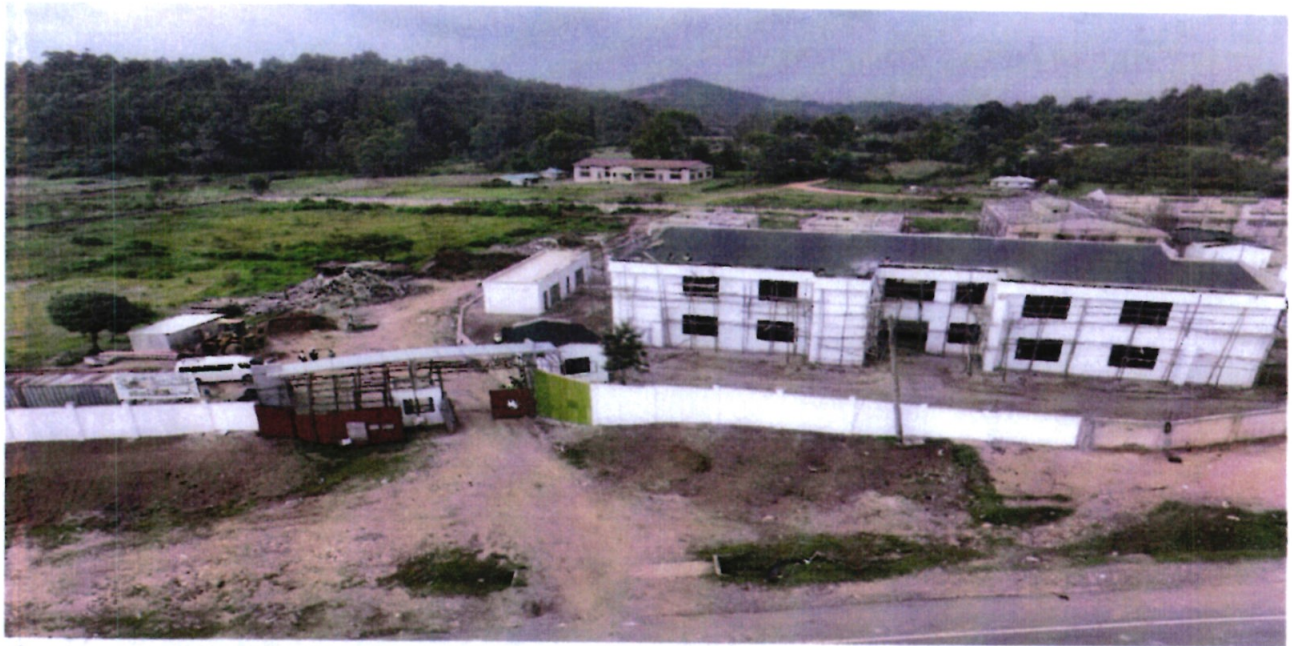
Ongoing construction of the Kshs 5.8 billion gold refinery at Lidambitsa area in Ikolomani constituency of Kakamega County.
