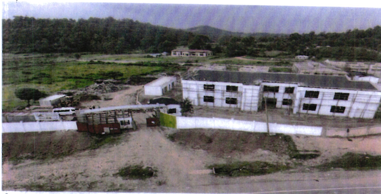
Ongoing construction of the Kshs 5.8 billion gold refinery at Lidambitsa area in Ikolomani constituency of Kakamega County.
