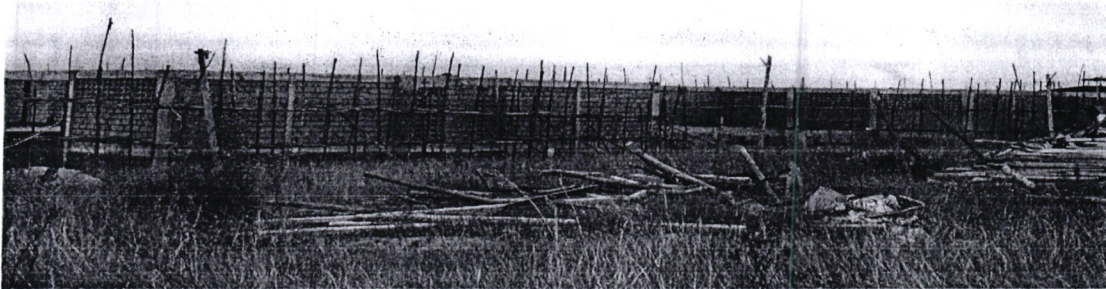
Front view of 4 small warehouses at 50% complete Overall the construction of the textile manufacturing hub is at 80% complete
