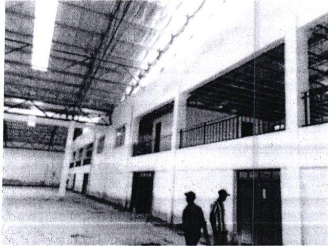
Internal view of the cluster, (Mezzanine) Railing and steel doors in place
