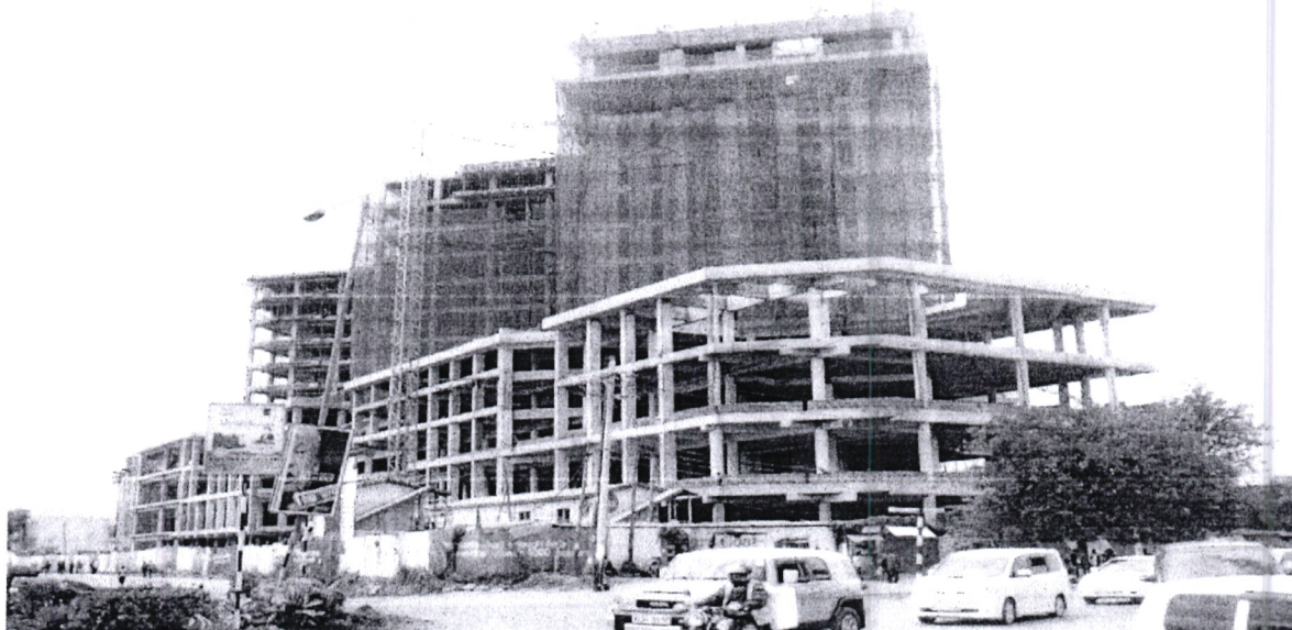
Research, Technology and Innovation Laboratories under Construction at KIRDI South B, Nairobi
