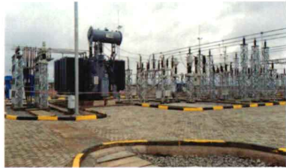
The power sub-station at the Naivasha SEZ
