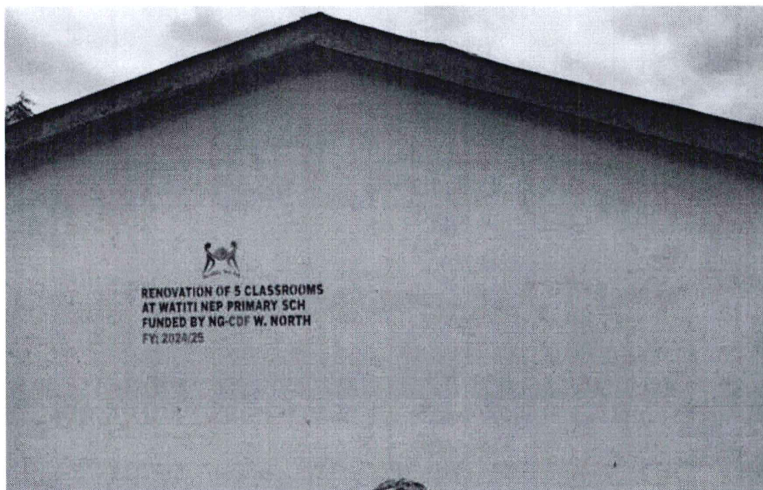
Watiti Nep Primary School: Renovation of 5 classrooms, (Reroofing, wall plastering, painting and flooring)
