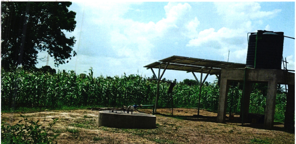
Solar Powered irrigation borehole at Chakama irrigation farm at Challa
