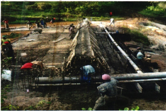
Gaitega Gaturi Small Holder project water intake structure and pipeline installation works
