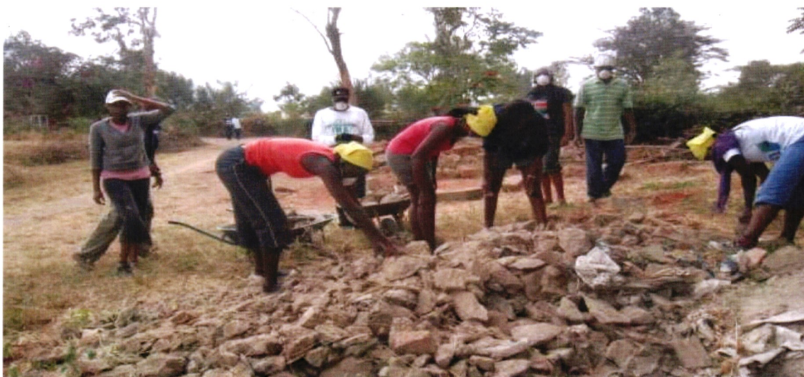
Award Participants from United State International University (USIU) preparing grounds for the construction of a classroom at Machakos Institute for the Blind. Over 50 projects are undertaken annually by different institutions across the country ranging from environment conservation, construction, awareness campaigns on youth development issues including conflict resolution and health care as well as contributing to the Big 4 Agenda.
