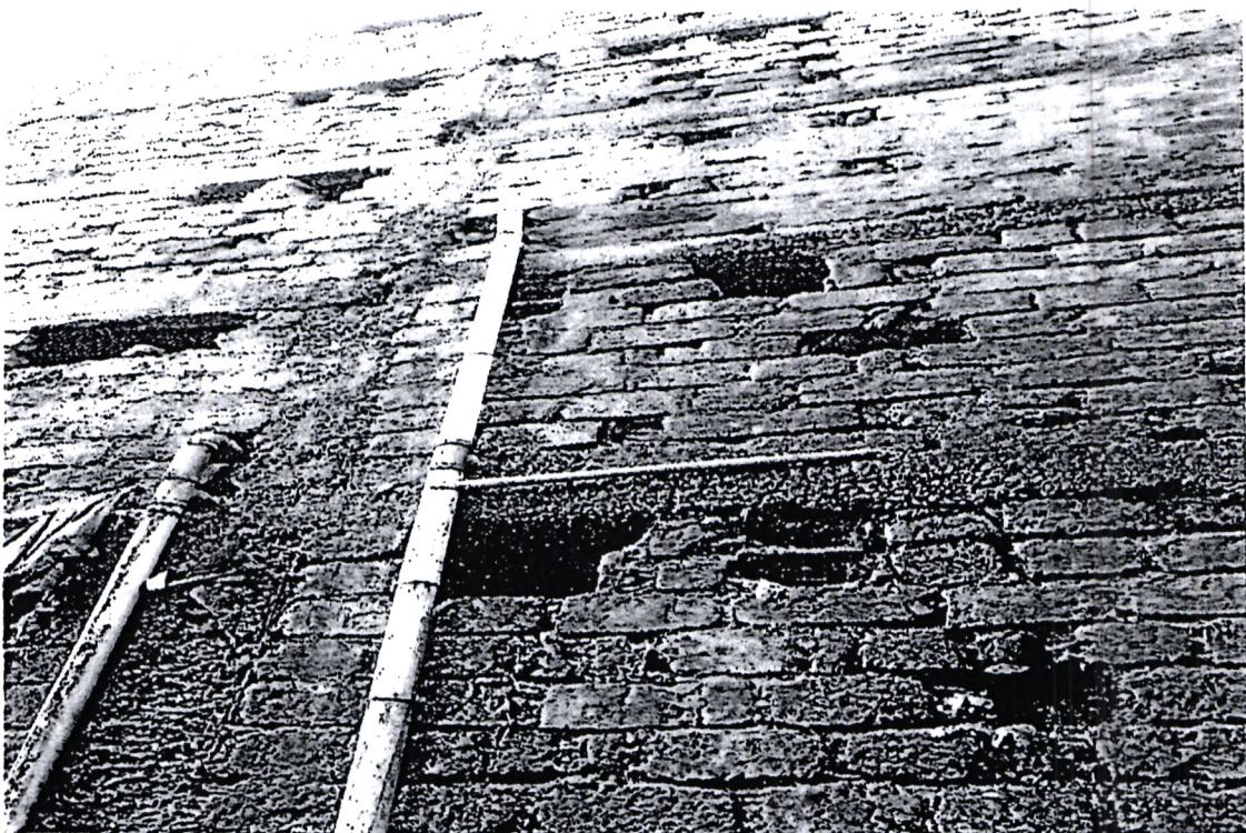
Plate 5: Elevation of Building Audited at Huruma, September, 2019. Failed the scientific tests and earmarked for demolition.
