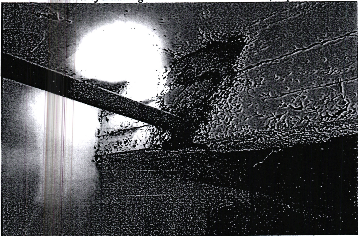
Plate 7: Cutting of beam to pass a waste water pipe thus compromising the structural integrity of the building.
