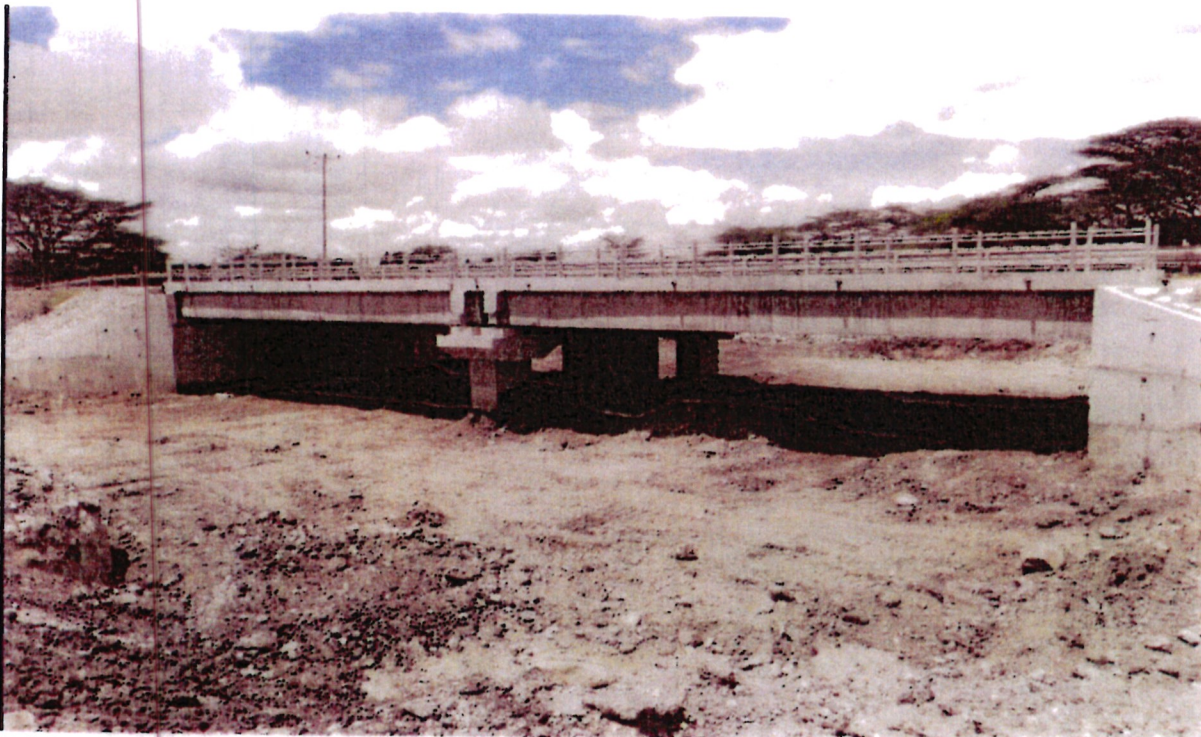
Widened 30m long two span concrete bridge at Km 36+093 along Kiserian – Isinya project corridor
