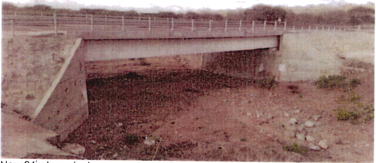
New 24m long single span concrete bridge at KM 18+743 along Kajiado – Imaroro project corridor
