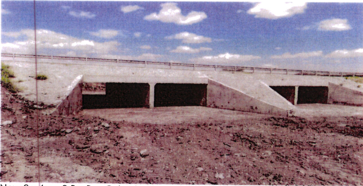
New 2 x 4m x 2.5m Box Culvert at Km 33+205 along Kiserian – Isinya project corridor
