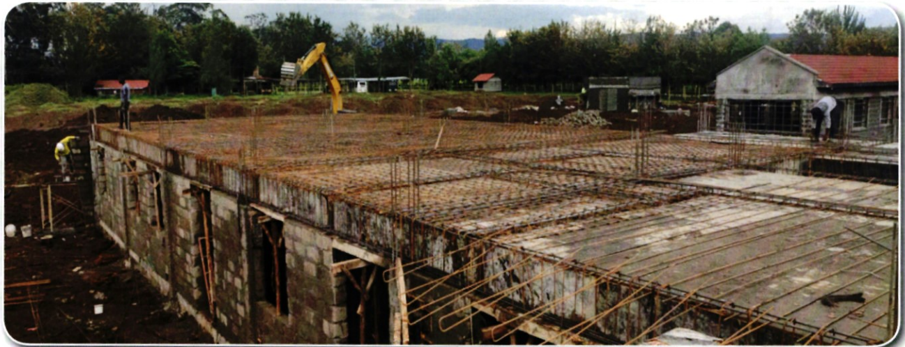
Ongoing construction of Lanet Regional Hospital at Lanet Barracks in Nakuru as at 30 June 2022
