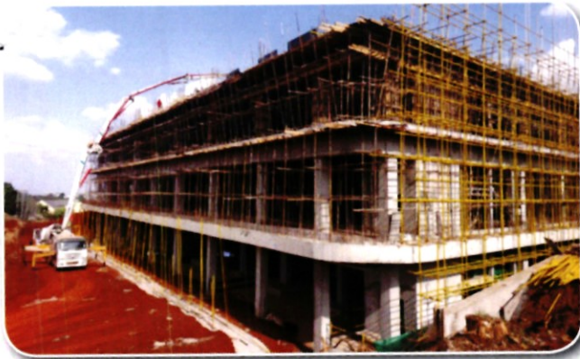
FRRH - Ongoing construction of Accident and Emergency Block at Kabete as at 30 June 2022
