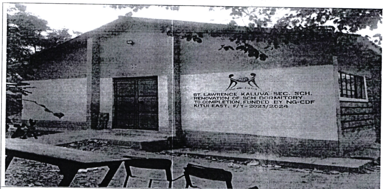
Fig. 1 St. Lawrence Kaluva secondary School – Construction to completion of 300 students capacity Dormitory
