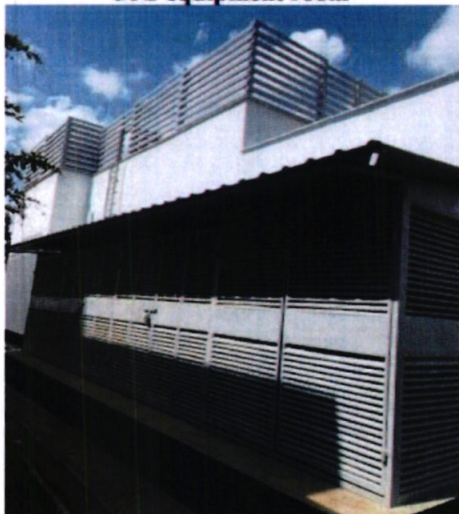
The side view of the bunkers building at UPS equipment room
