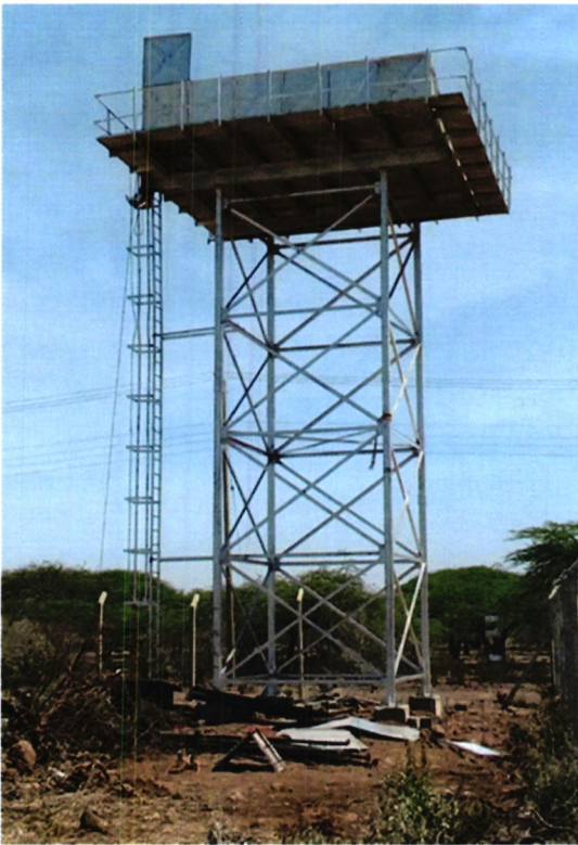
One of the elevated Steel Tanks for wat 1
