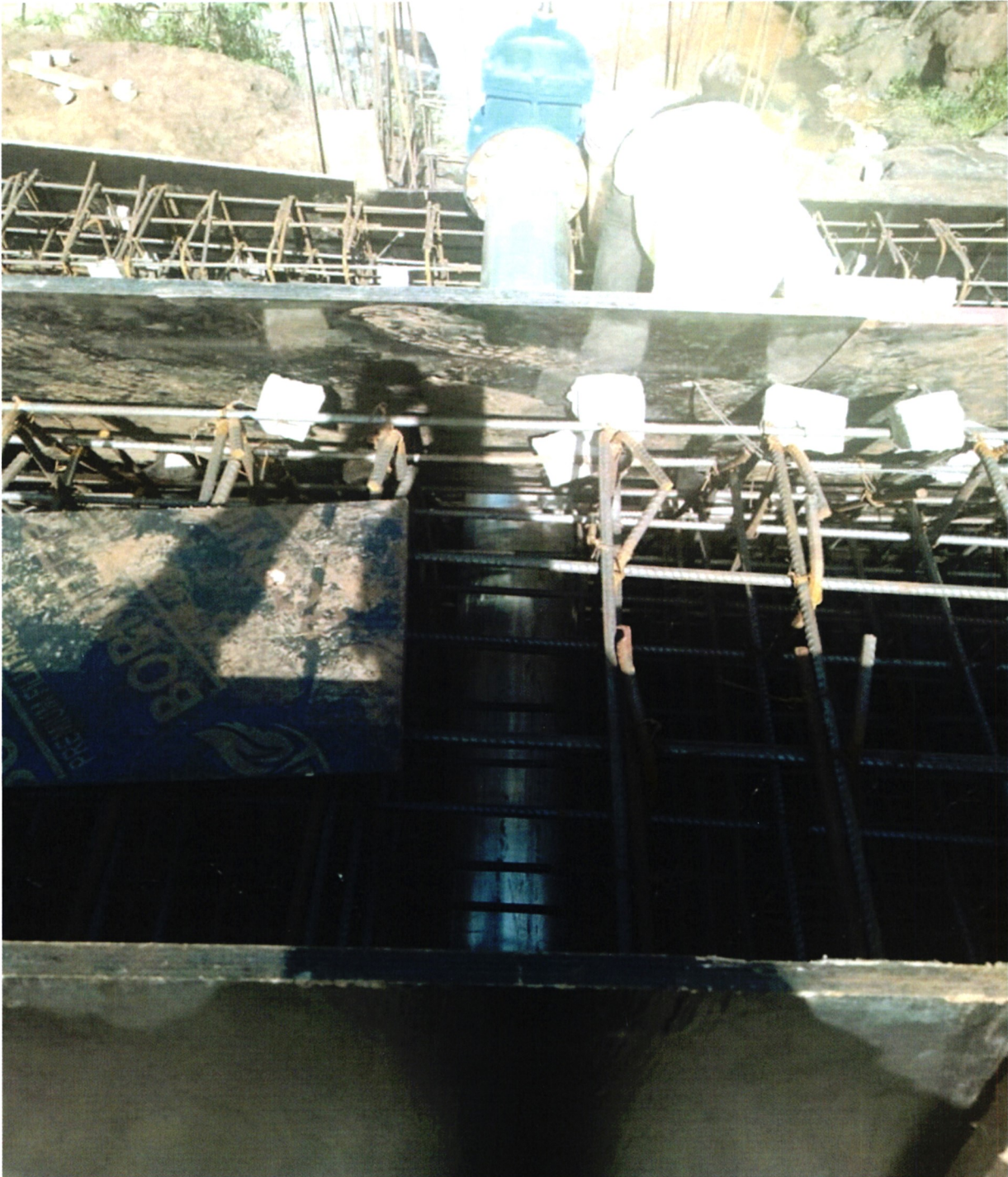
Figure 47: Gaitega Small Holder project water intake piping and reinforcement fixing works ongoing
