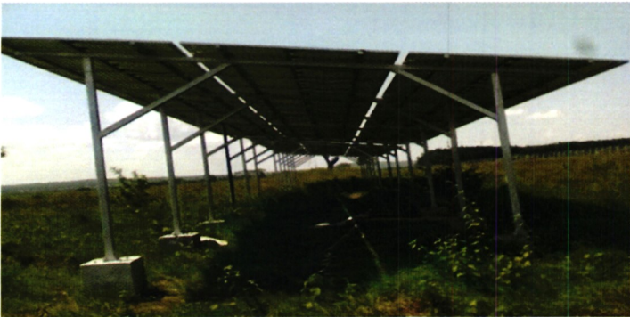
Solar panel array in Alupe
