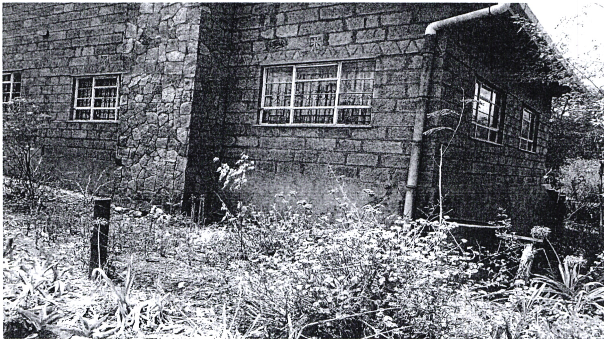
Figure 3: A house that was affected by the blasting of rocks in the path of the railway with cracks appearing in the houses on 26.4.2019. (Kajiado County)
