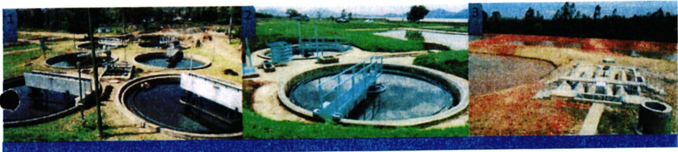
Picture 10: The Completed rehabilitation of Kisumu (1), Homa Bay (2) and Bomet(3) Sewerage treatments facilities in Kenya
