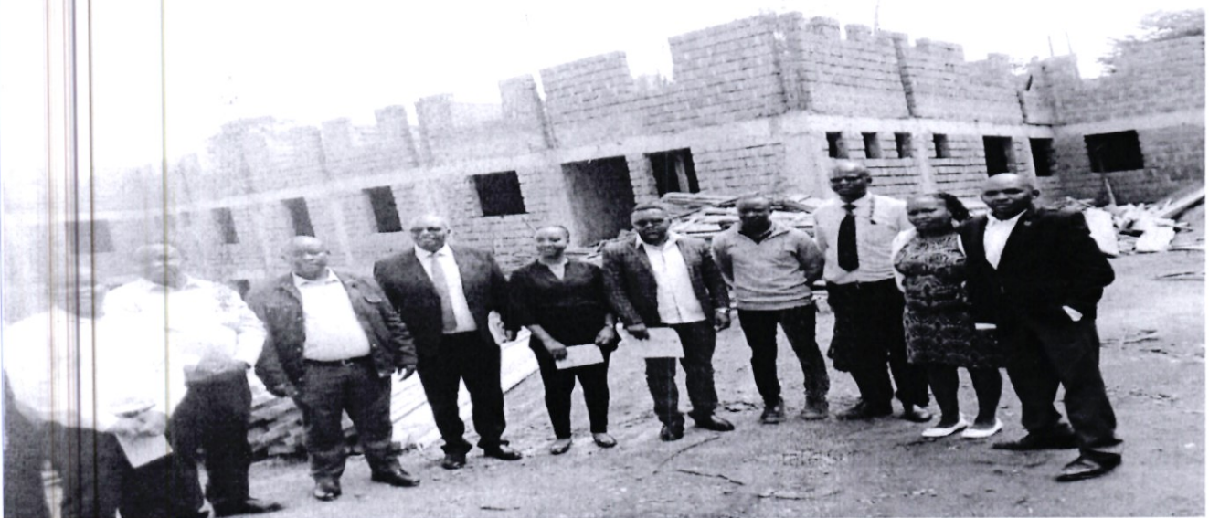
Front section of the Safe House for NGAAF in Nairobi County. The structure awaits roofing (some roofing materials on site), finishes, mechanical and electrical and civil works
