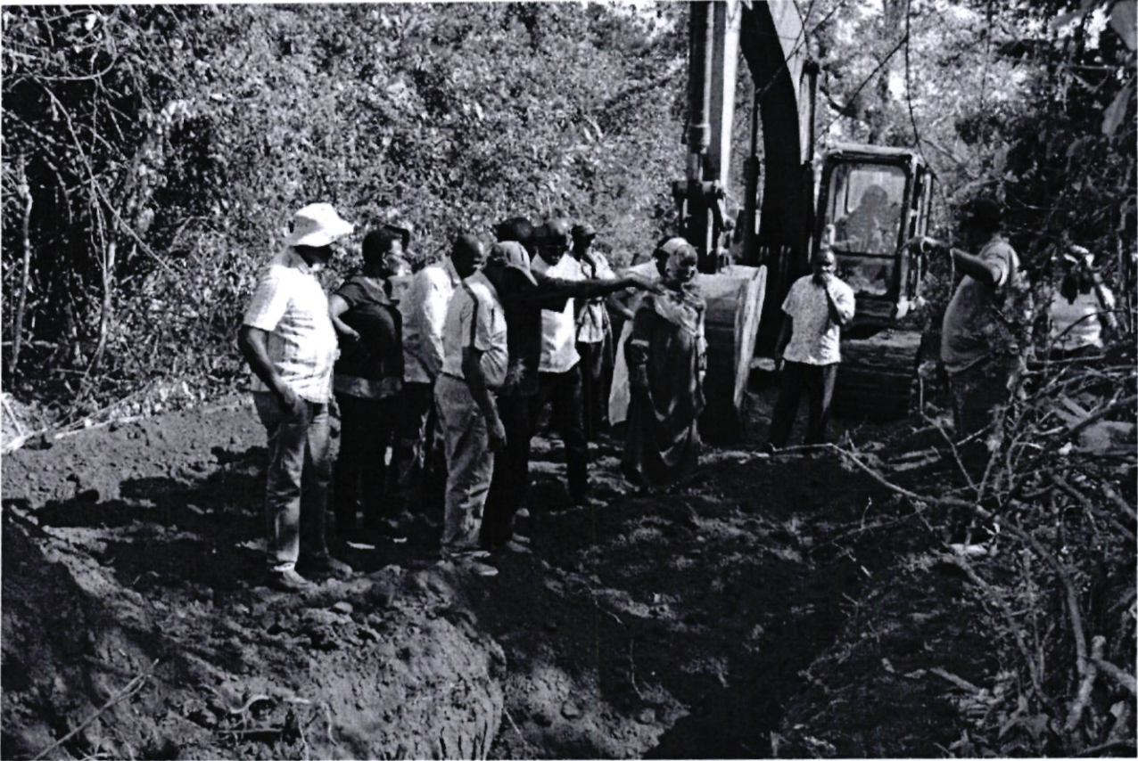
Board of Directors inspect the laying of pipes for Nyaru water project in Kirinyaga County
