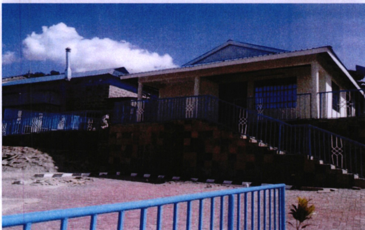
CWSK integrated child and family centre in Murang'a – Work in progress: House blocks 1&2 (above), health centre, guard house and parking complete (below)
