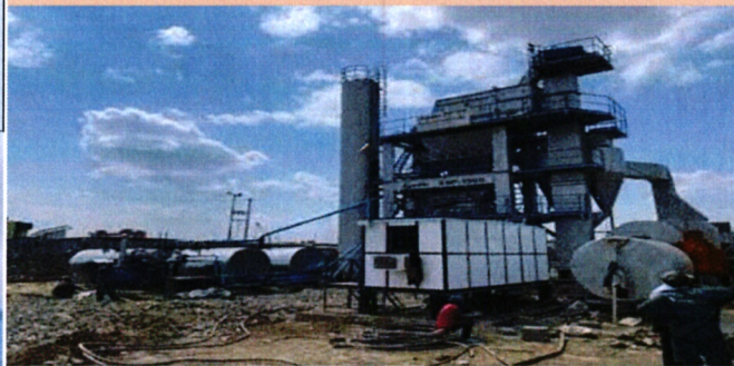
Asphalt Plant Constructed in Kangundo by NMS used for processing bitumen and asphalt
