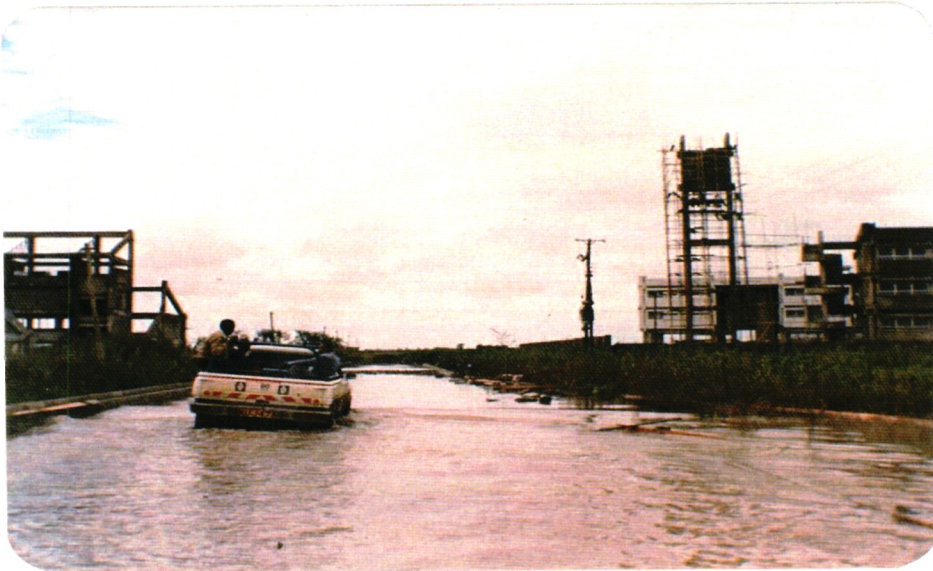
A Construction site photo of KLB headquarters in South C taken on May 12, 1989
