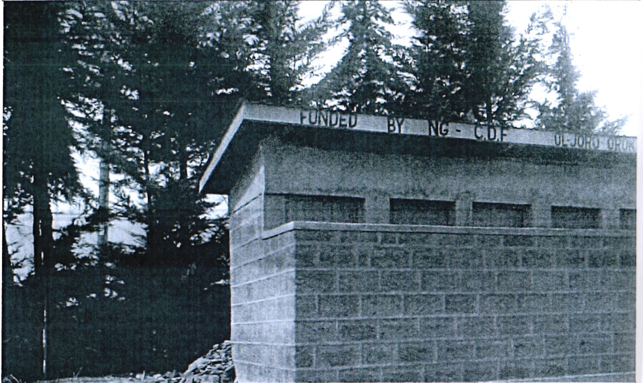
Due to shortage of pit latrines, we constructed several latrines e.g the above diagram of Muchemi Primary School
