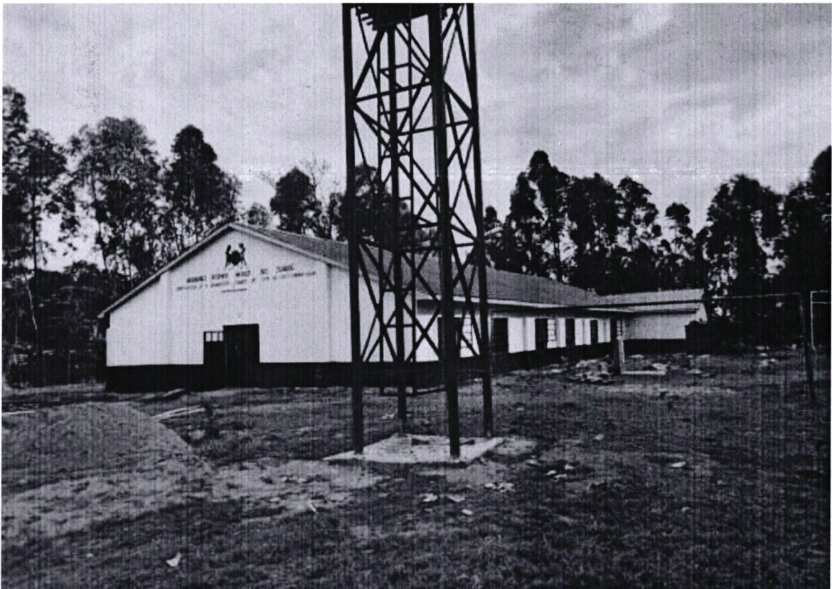
CONSTRUCTION OF A DORMITORY AT ARGWING'S KODHEK FUNDED BY GEM NG-CDF IN THE FINANCIAL YEAR 2018/2019 -2020/2021
