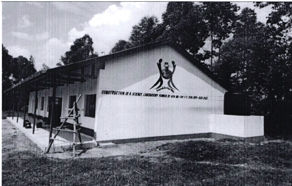
CONSTRUCTION OF A SCIENCE LABORATORY AT YALA TOWNSHIP SECONDARY SCHOOL FUNDED BY GEM NG-CDF
