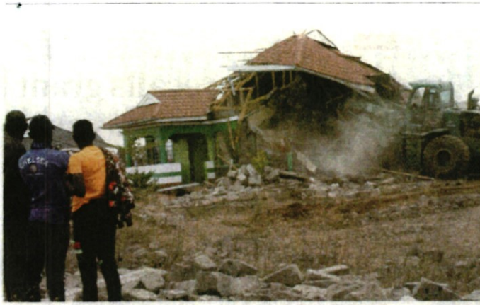
A bulldozer demolishes a house on land that belongs to the East African Portland Cement Company in Athi River on Monday. [Peterson Githaiga, Standard]
