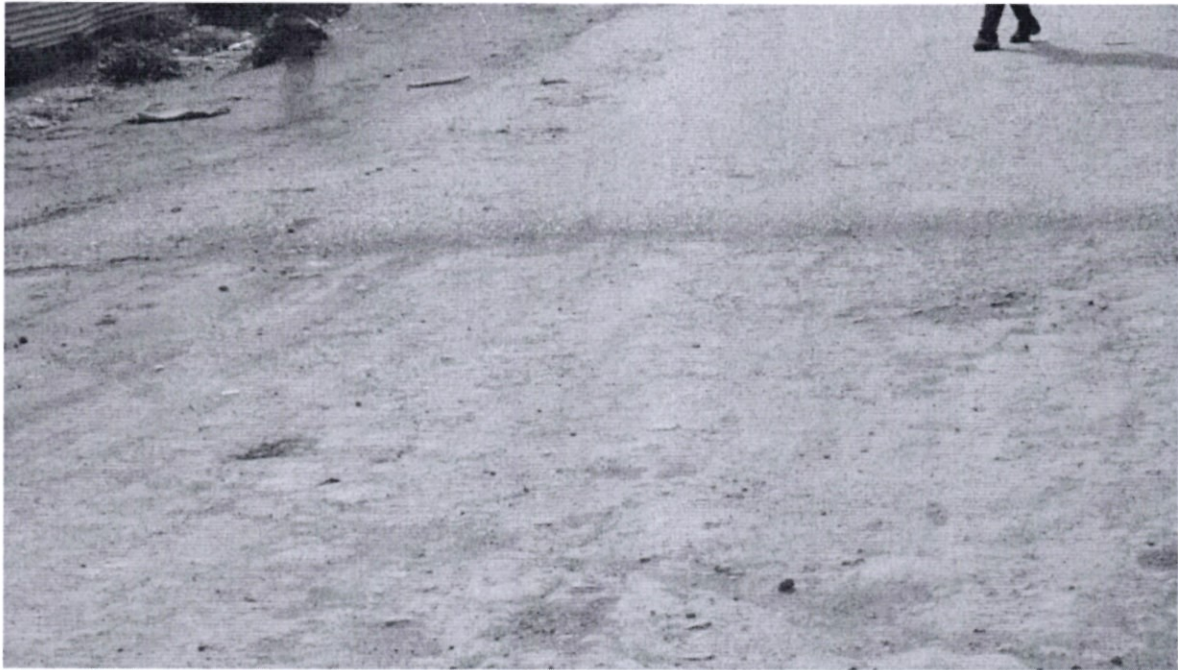
Figure 3. A section where the tarmacking of the road stalled
