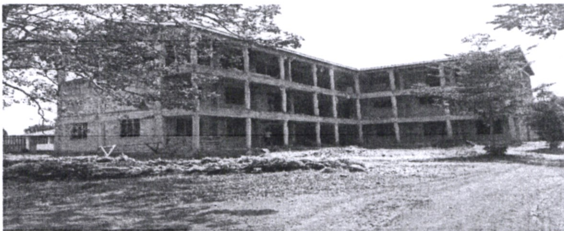
Khwisero Girls' Secondary School - Construction of a storey building comprising of Administration Block, 1 no.classroom, Computer Laboratory and Library. The school is funding an extra floor. The project is ongoing.
