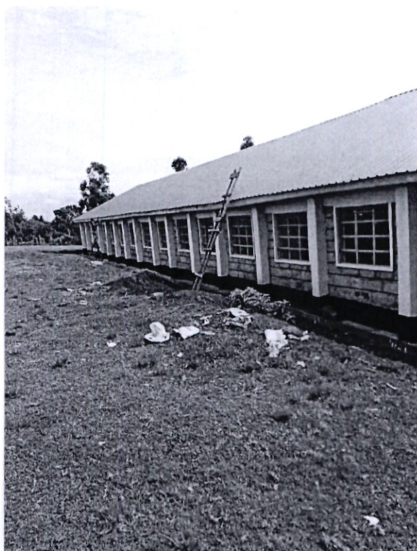
KEBULONIK PRIMARY SCHOOL CONSTRUCTION OF 8 NO CLASSROOMS Implementation challenges and recommended way forward
