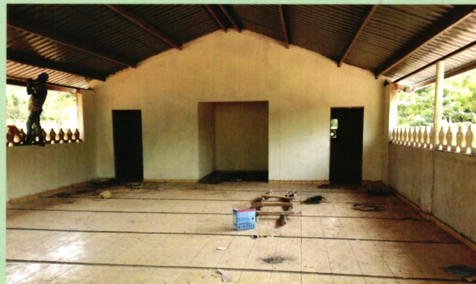
Manyani Camp Mosque under construction inside the Manyani Prison. This will serve close to 400 Muslim inmates. Ummah Foundation is the sponsor of this Project.
