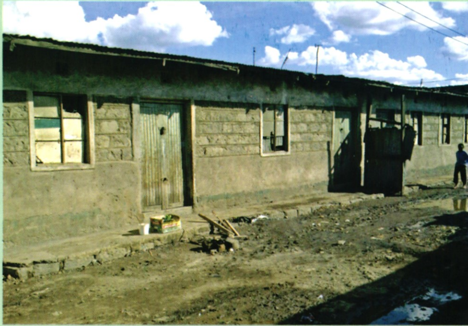
The dilapidated Madrassah classrooms that need to be renovated and be put into proper utilisation by more than 100 students of Soweto slums.
