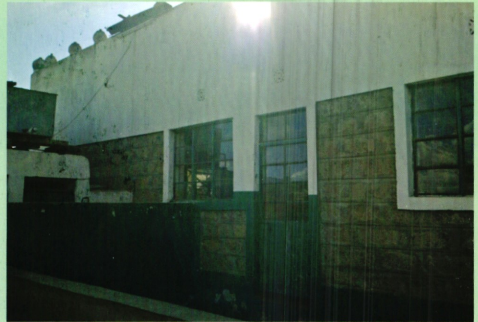
Part of the Soweto Mosque Project that is earmarked for renovation and rehabilitation. The Mosque is in the Soweto slums that has a population of about 780,000 people and the infrastructure is very poor owing to the fact that the area has been relegated for many years. The Muslim population stands at around 1000 and the population is growing every day. Within the coming years the mosque won't be able to accommodate the number of worshippers. Ummah Foundation is teaming up with well wishers to renovate the mosque, rehabilitate the 3 classrooms for the Madrassa and the upgrade the Imam and teachers quarters.
