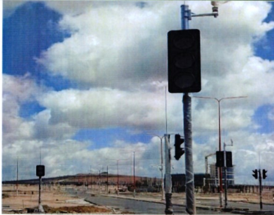
Traffic light poles installed in the city.
